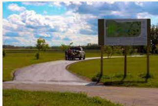
A worker applies the finishing touches to the newly paved portion of path on Logan Green (OFF, 2022).
