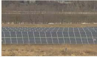
The solar array in Lumsden is the size of two football fields (ODLUM, 2022).
